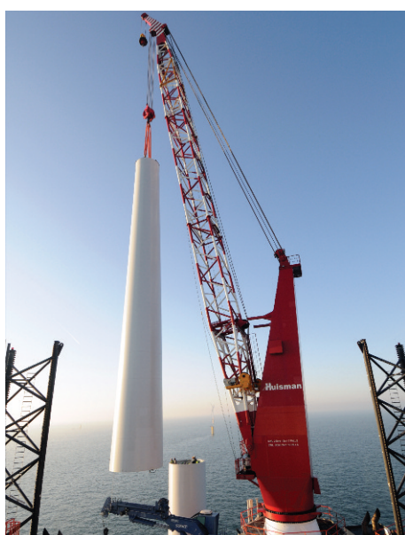
The lead operator(s) will be responsible for the construction of the wind farm projects. Photo by CHPV courtesy of Scira.
